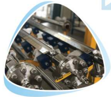
Instrumentation – Level, Pressure, Flow
