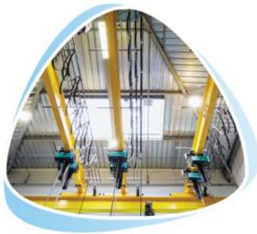
Electric Winches and Hoists
