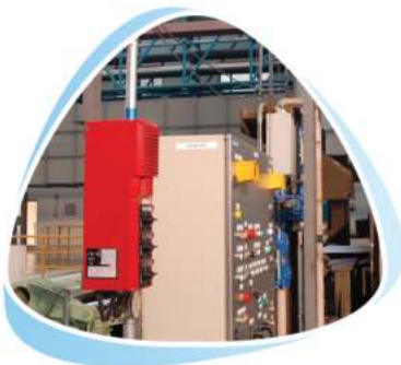
Public Address General Alarm (PAGA)
