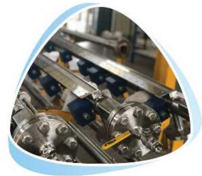
Instrumentation – Level, Pressure, Flow
