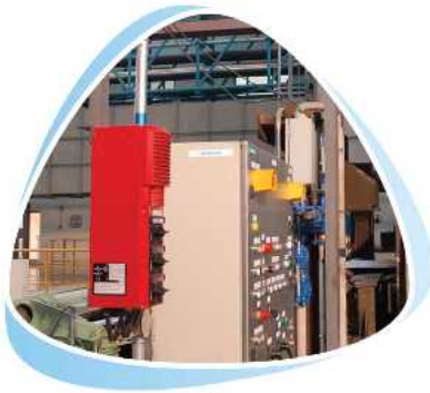
Public Address General Alarm (PAGA)
